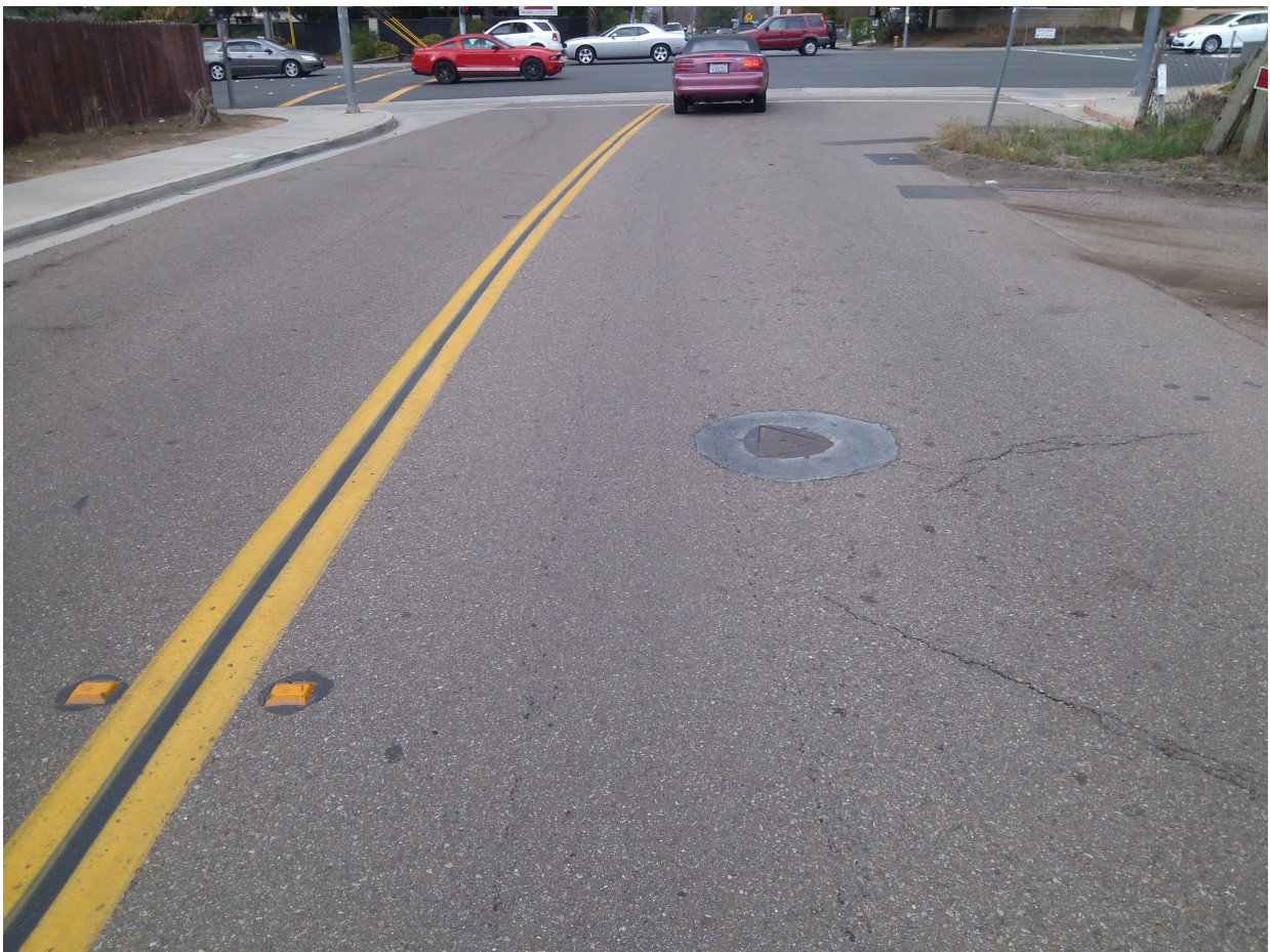
Illustration 8: Note that there is a survey Monument designating logical center of the street (edge of El cajon) but it is far from double-yellow lane marking. If lane marking were moved to this monument, then there may be enough room for parked cars and a traffic lane. But it looks like then, there is not enough room on the other side.
